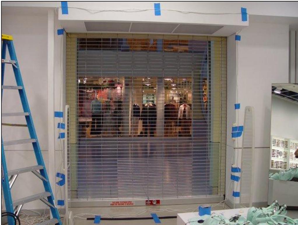
Figure 1. Installation Ready for Tuning
